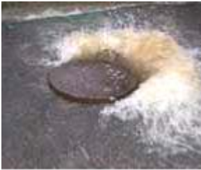
Sewer Network Flooding
