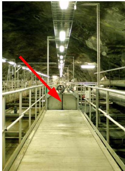
Aeration basin inlet channel with control hatch (red arrow)
