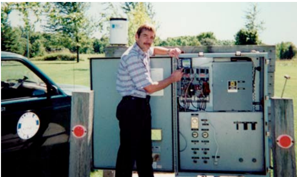
Bruce Neerhof at Kohler's Pump Station Monitor.
