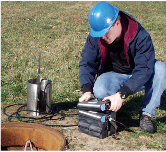
Figure 3. Quick, simple setup and deployment are popular features with field crews.
