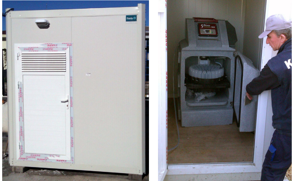
Teledyne Isco 5800 refrigerated sampler installed at an industrial outlet
